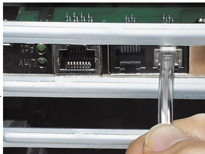
Standard phonenumber cabling with RJ-11 tips
